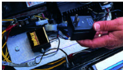
(Top left to right) Officers of the Arlington, Texas police Department using PulseTech to ensure battery performance on their bikes. (Bottom) The RediPulse 6-12 installed on a motorcycle.
