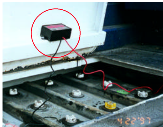
(Top) CSXT installed two 36-Volt PowerPulse units (bottom) on their locomotives to improve battery charge acceptance and overall performance on the 72-volt battery systems.
